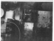
Portable transformers are used in light engine plants required to be built.
