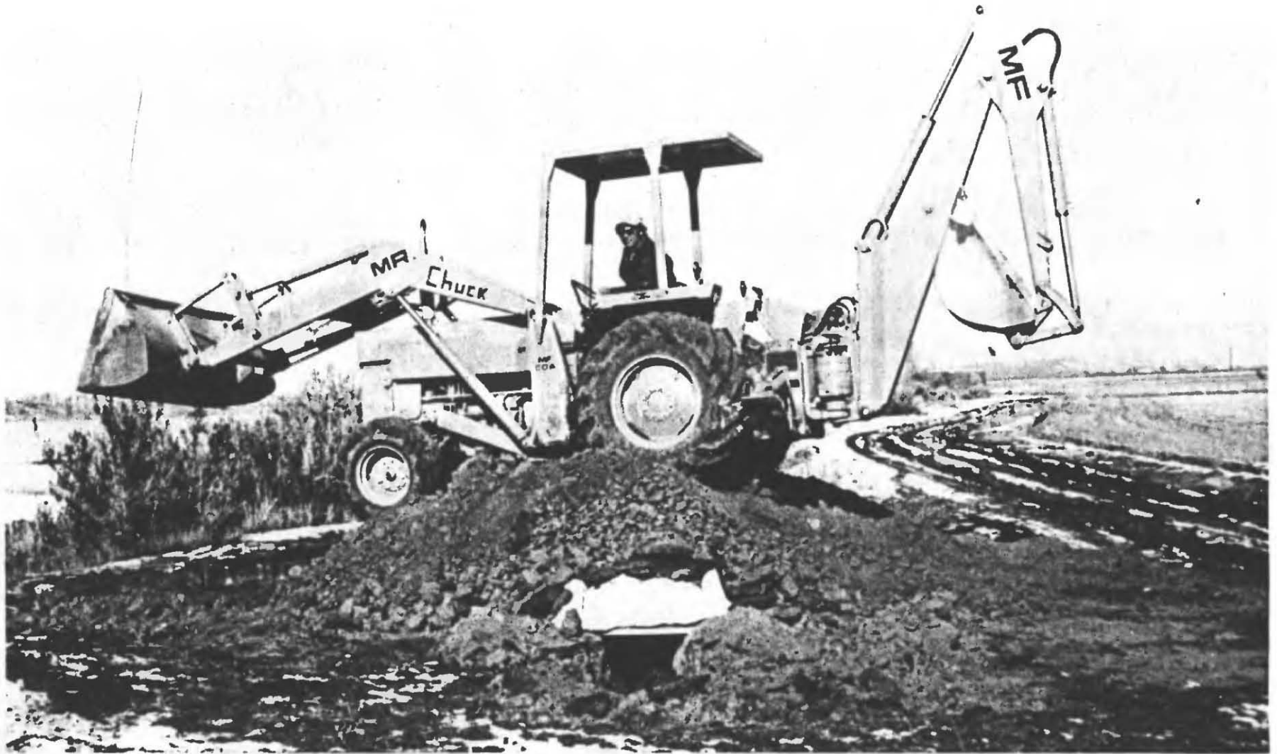
Fig. 3.3. An 8-ton backhoe on top of what was originally the 6\frac{1}{2} -ft-deep pile of earth over the shelter. Before this picture was taken, this machine had been driven back and forth several times over the mounded earth. The roofing doors remained undamaged, and were not observed to be bowed downward any more than when only the 6\frac{1}{2} -ft mound of earth was over them.
