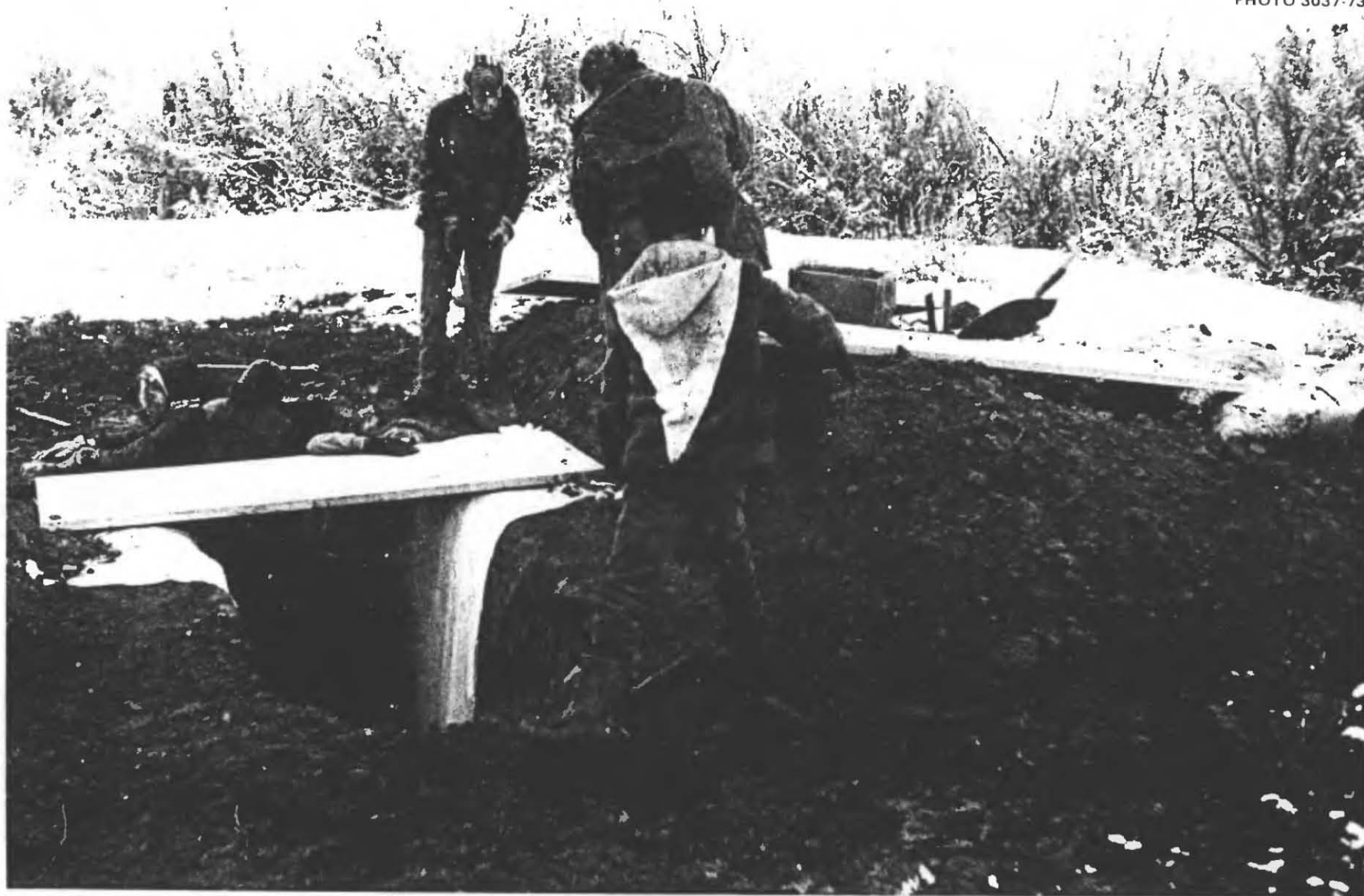
Fig. 2.9. Placing the first of six interior, hollow-core doors over the completed trench. The earth on the wall-lining sheet was removed before the second door was positioned.
