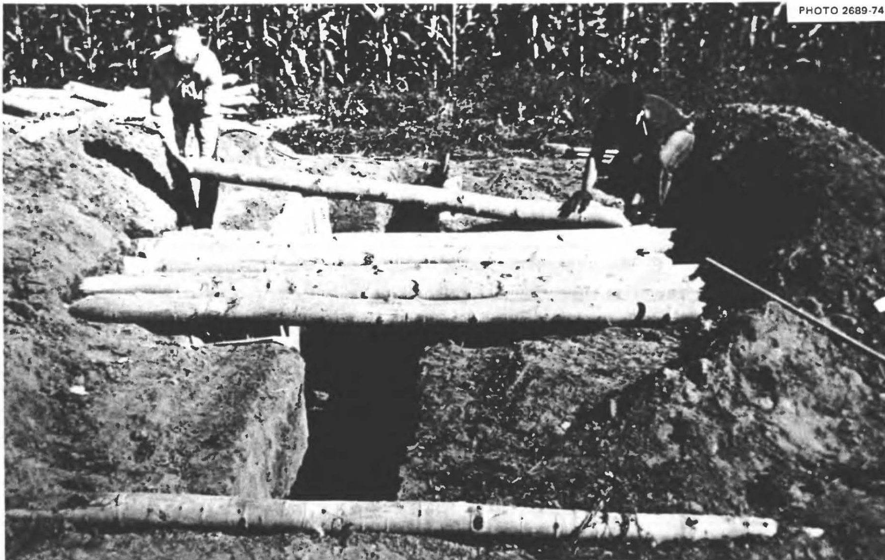
Fig. 4.7. Placing the 9-ft roof logs, all 2 ft off center, over the 3\frac{1}{2} -ft-wide main trench. A shelter in firm earth such as this, with 9-ft roofing logs positioned 2 ft off center, would enable the builders to widen their shelter to a 5\frac{1}{2} - or 6-ft width and to deepen it to standing height. If their home and community were destroyed, the family could live in such a rainproof dugout for months, if necessary, while minimizing their radiation doses and being more comfortable, in cold weather, than if living in a tent or shack.
