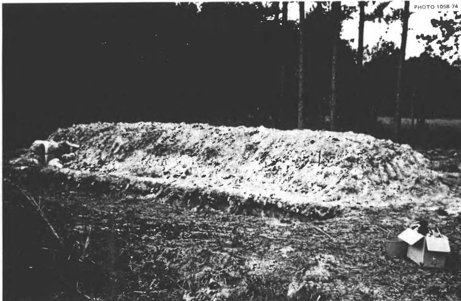
Fig. 5.9. The completed shelter, after a full 15 in. of heavy, wet, sandy earth had been piled on top of the roofing doors. These doors had all been painted or varnished with two coats, to simulate the interior doors from an average home. As an additional means to keep dampness from weakening the cardboard honeycomb inside these hollow-core doors, the walls made of earth-filled rolls were made about 3 in. higher on one side than on the other. Then waterproof materials (shower curtains, plastic film, and plastic clothes bags) were placed directly on these sloping doors. Finally, earth was piled 15 in. deep on top of these waterproof door coverings.
