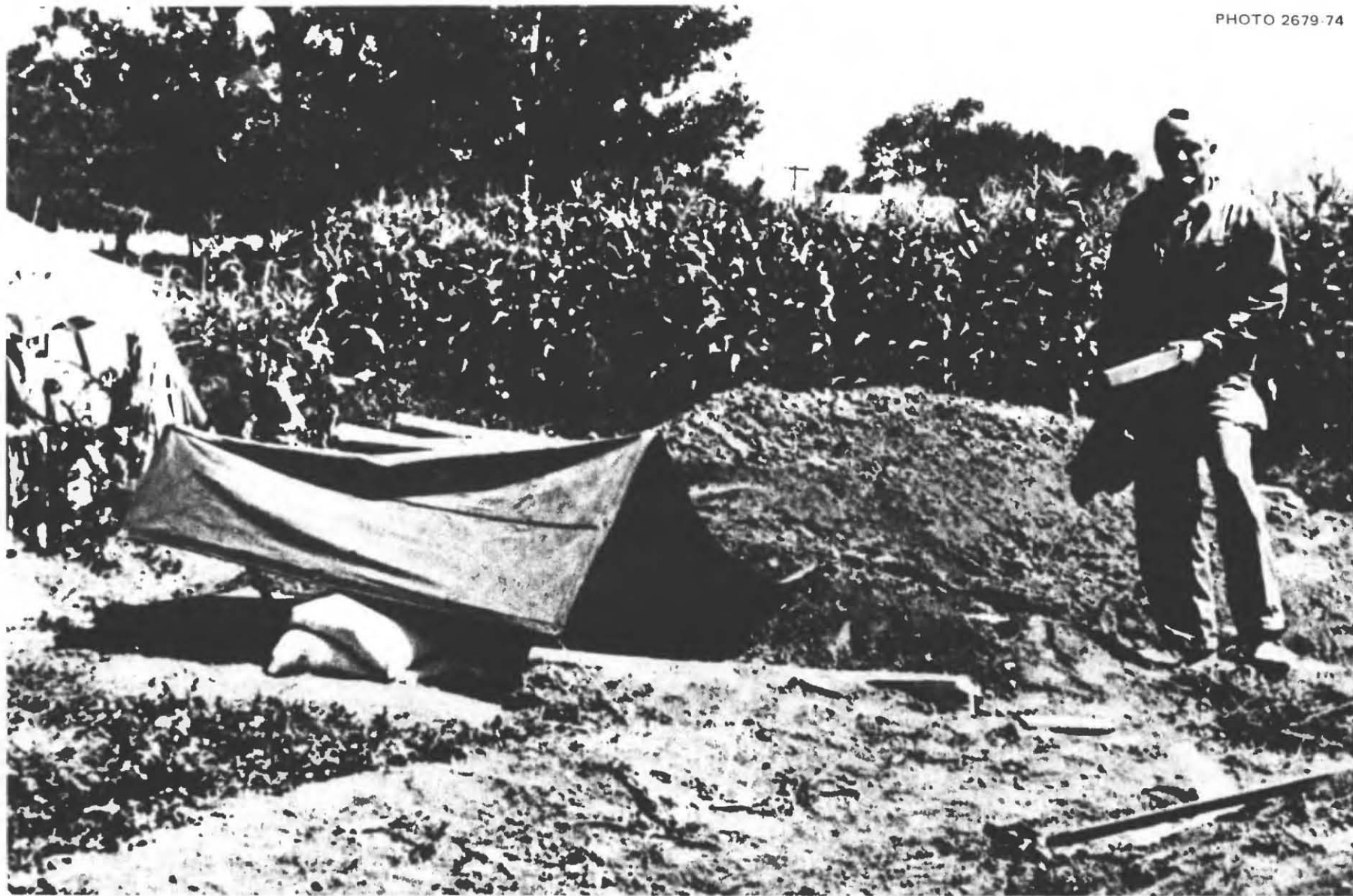
Fig. 4.11. Outside the completed shelter, with the family of six – and their dog – inside. Thirty-two and one-half hours elapsed from the time this family received an Evacuation Check List and the shelter-building instructions at their home in Bountiful, to the hour they completed their shelter near Spanish Fork and began the continuous occupancy test.
