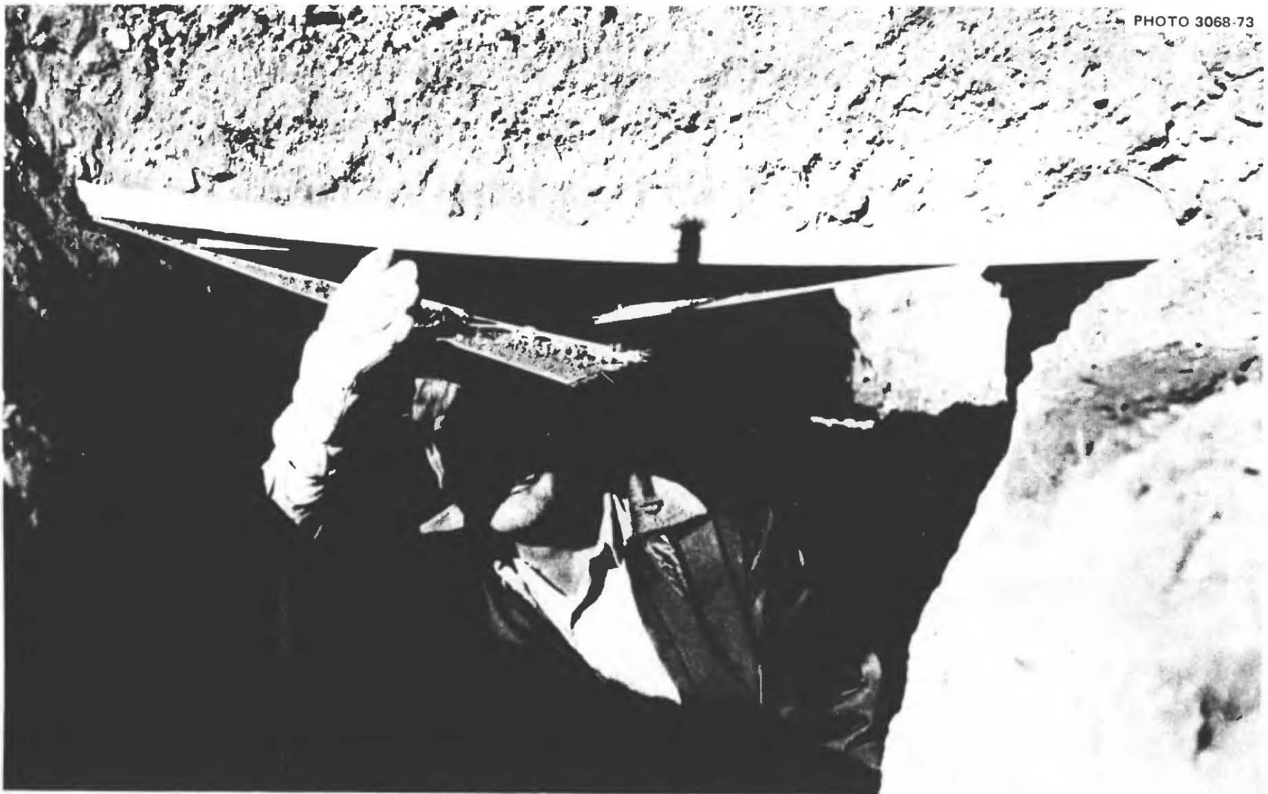
Fig. 3.9. View of the most damaged door after the removal of the adjacent door. Removal of some of the weight on the 1\frac{1}{2} × 1\frac{1}{2} -in. pine board that formed the unbroken frame of this door resulted in its becoming less bowed. The dry-earth bank pictured above this door appears to be vertical but actually was not. Kearny concluded that all that is needed to build a blast shelter in areas with stable and adequately deep earth is: (1) a deformable membrane (such as a tarp or rug) strong enough to support the weight of earth between it and the bottom of the earth arch formed by downward stresses and strains in the earth above the membrane; (2) the earth itself plus some practical although uncommon knowledge of how to use merely such a deformable membrane and earth to build a blast-protective roof over a trench.
