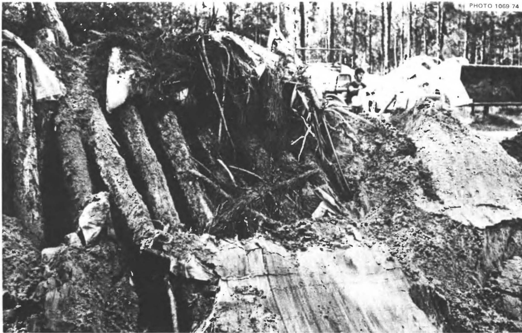
Fig. 5.40. View after a backhoe had started to demolish the Waldens' Ridge-Pole Shelter, which proved to be decidedly sturdy. Note that some of the wall poles were broken before they were moved off the ridge poles, or the ridge pole had been moved significantly.
