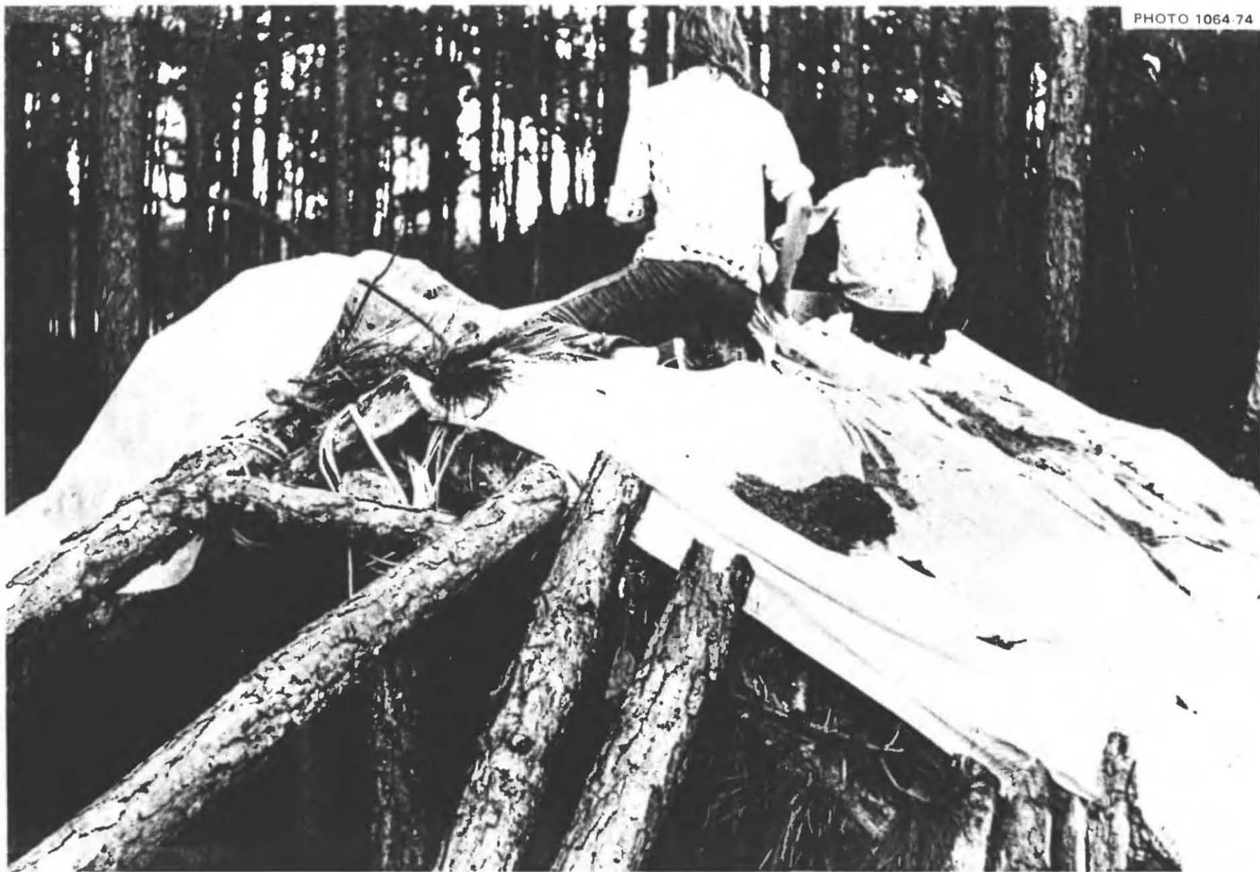
Fig. 5.34. Placing bed sheets over the pine limbs that had been placed crosswise over the roofing poles of the shelter. After the whole shelter had been covered in similar fashion, earth was shoveled or carried so as to cover the entire shelter. This covering was done from ground level upward.
