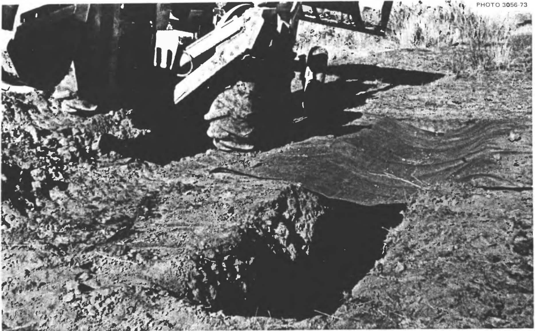
Fig. 3.12. Compacting the earth over one edge of the tarp. This edge has been placed in one of the two 16-in.-wide by 12-in.-deep rectangular trenches, each of which was dug parallel to and 3 ft from the vertical walls of the shelter trench. Packing with this wide-wheeled backhoe did not compact the earth as well as hand-tamping it with a pole.
