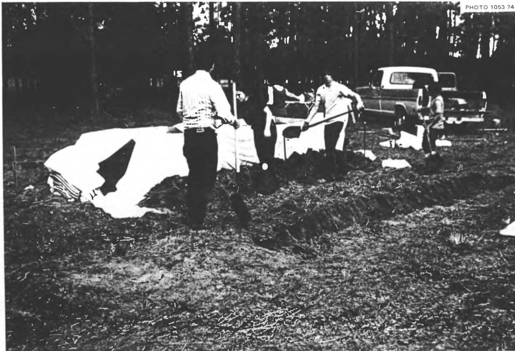
Fig. 5.4. Starting to make the first roll by shoveling earth onto bed sheets that had been placed with 2 ft of their long sides on the ground, with the rest of the sheets temporarily draped over the doors used as forms. This sandy earth could be dug quite easily with shovels.
