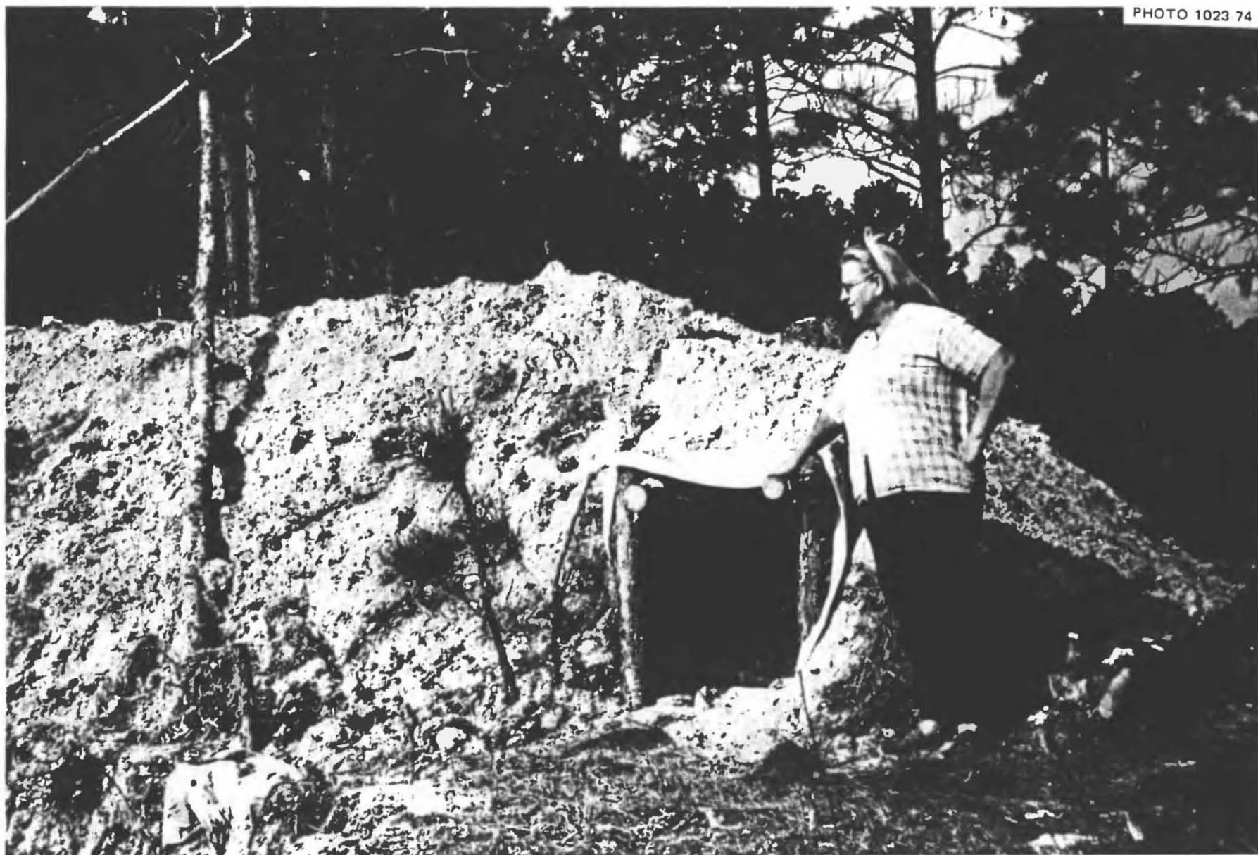
Fig. 5.52. The properly completed entryway of the A-Frame Pole Shelter, pictured on the day following its completion. These hard-working rural families built this 21-person shelter in 12 hours 14 minutes, from the time they received the instructions on a farm about 2 miles from the shelter-building site.
