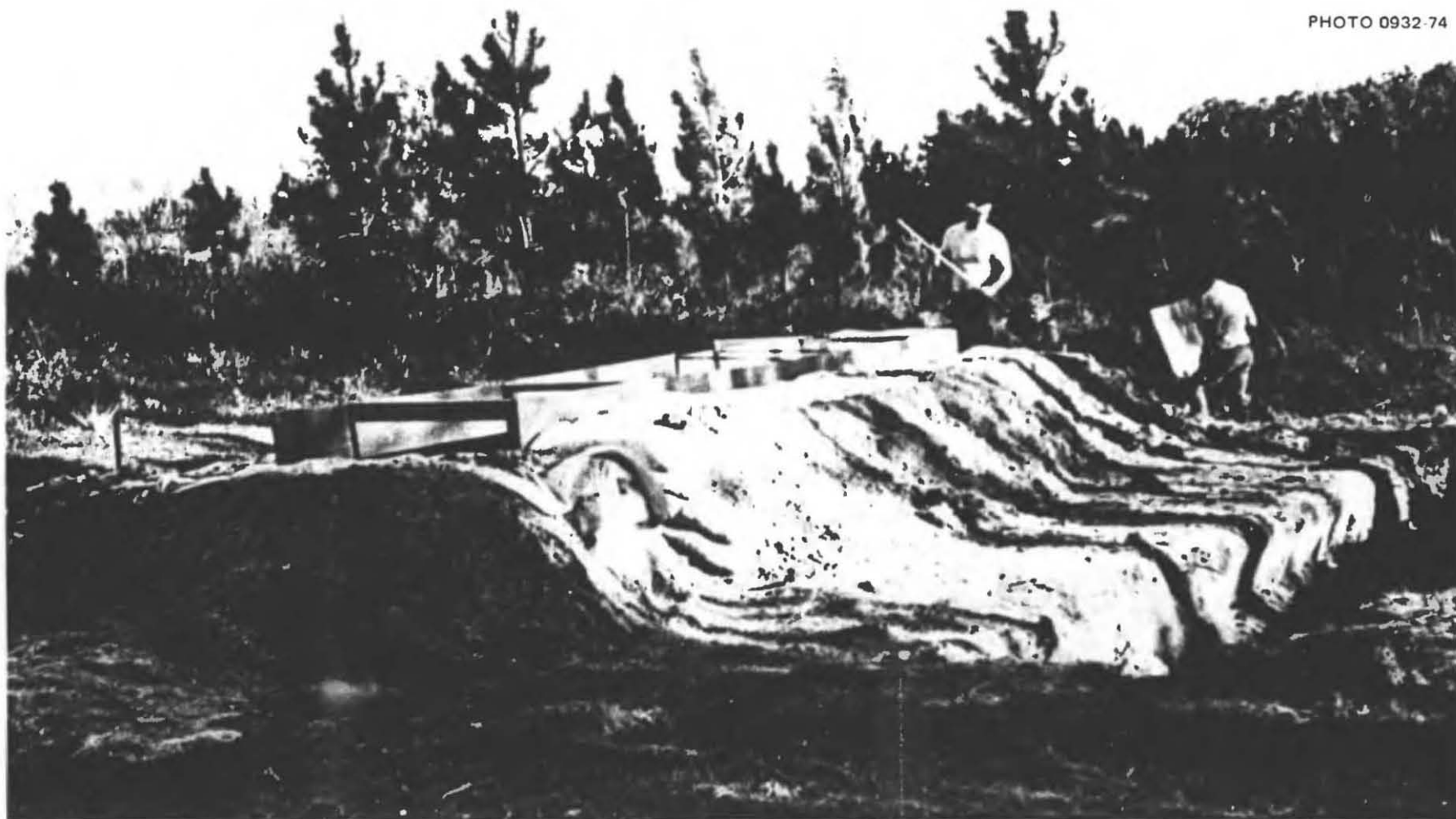
Fig. 5.7. One of the side walls, made of three rolls placed one on top of the other, pictured shortly before the door forms were removed.
