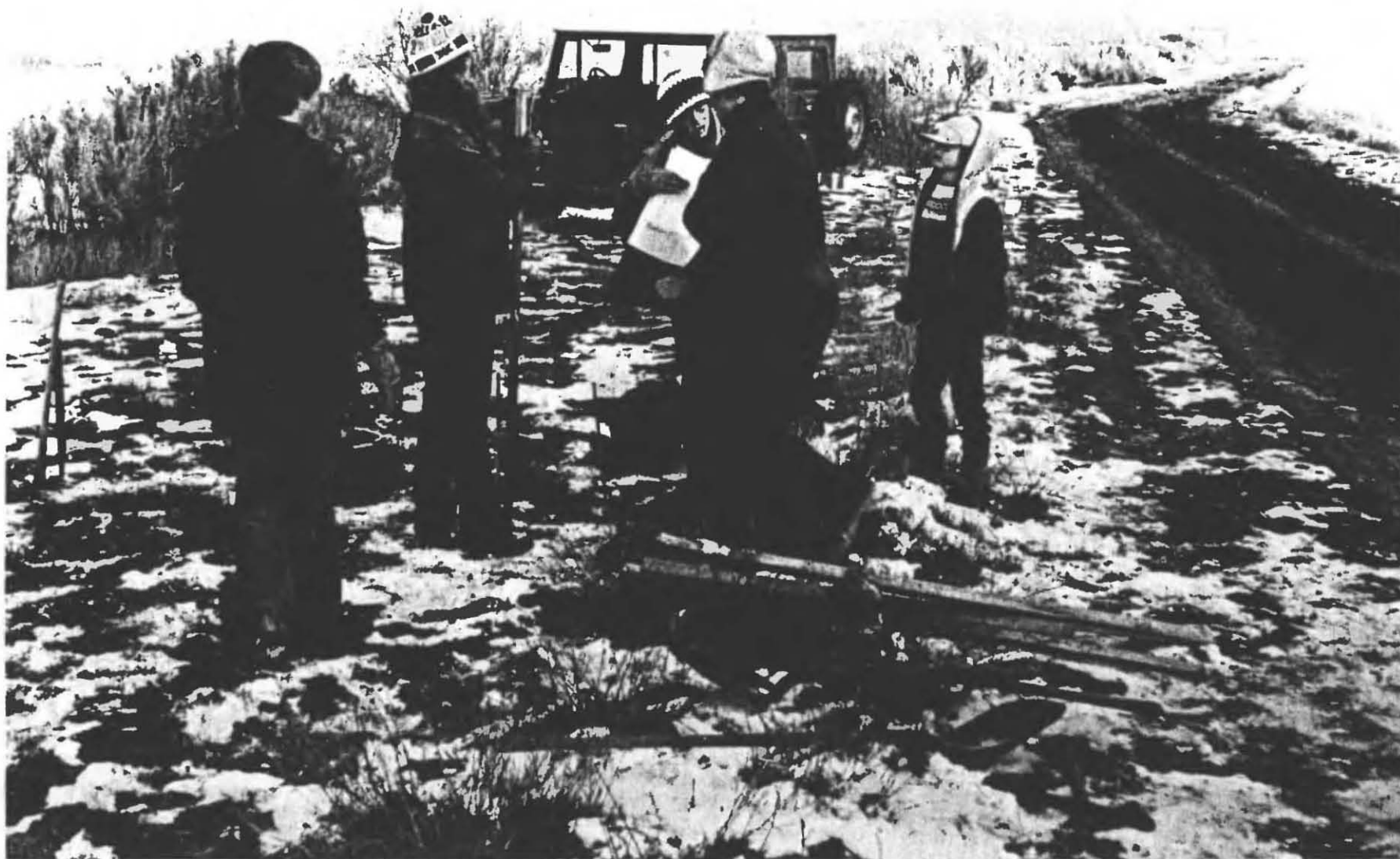
Fig. 2.2. Starting to stake out the shelter trench near Montrose, Colorado, at 7:17 AM. The six doors, some tools, water, etc., were carried in a station wagon. The ground was frozen only about an inch deep.
