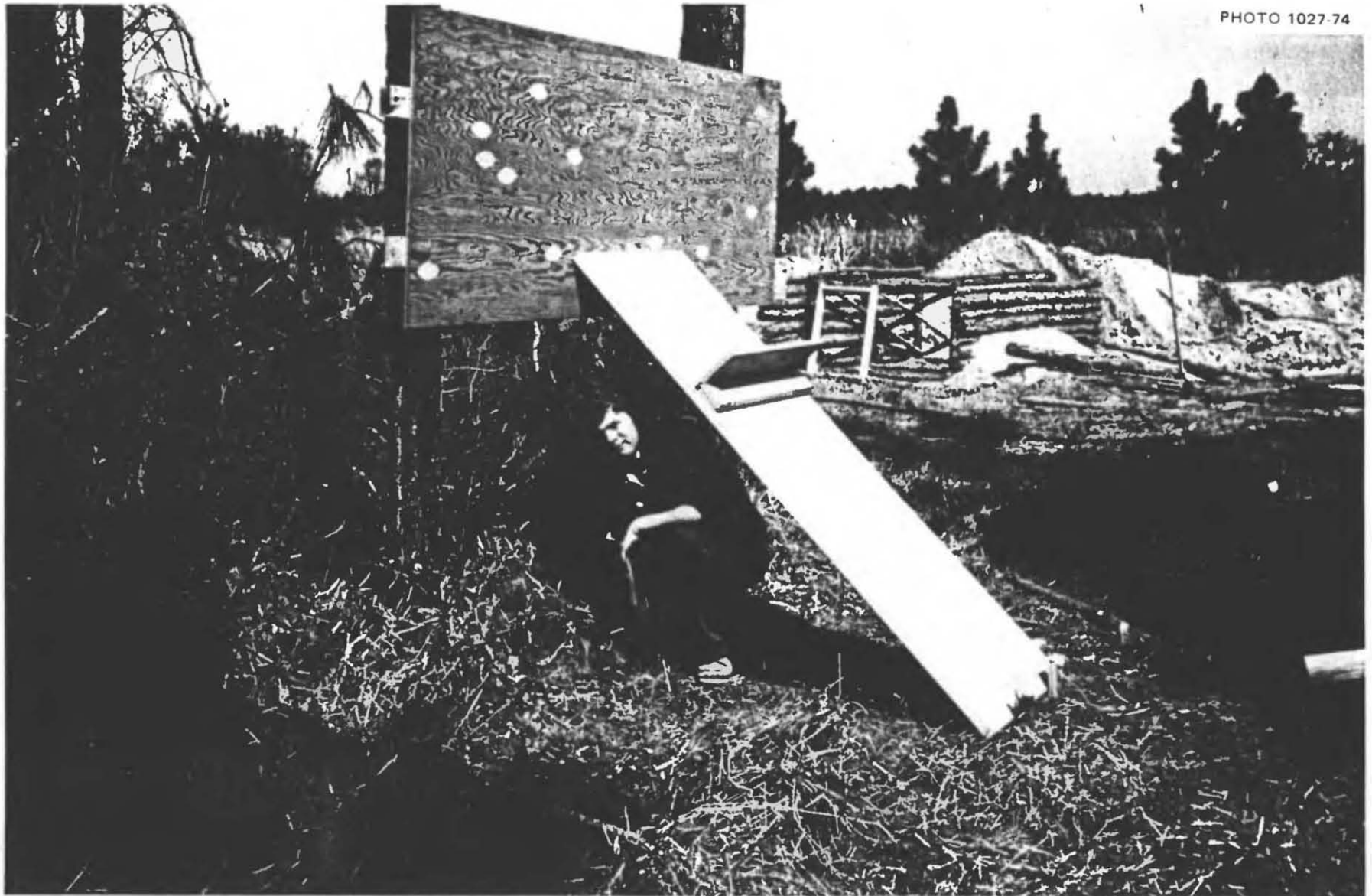
Fig. 5.63. Preparing to test a hollow-core interior door used as a roof door of an expedient Tilt-Up Shelter, built following instructions received from Donald A. Bettge, DCPA. The plywood (that was nailed to the horizontal 2 × 4s connecting the two pine trees) represented the side of a house. The door slopes 45° and is secured at its base by stakes.
