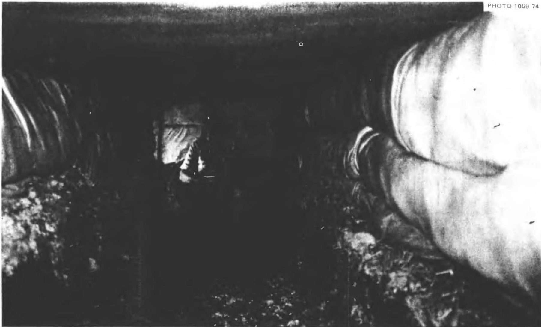
Fig. 5.12. Interior of the shelter, showing the roofing doors sloping from the right to the left, and bowed downward about 1 in. due to the 15 in. of wet earth covering them. This bowing occurred as soon as the doors were covered and did not increase during the following days.
