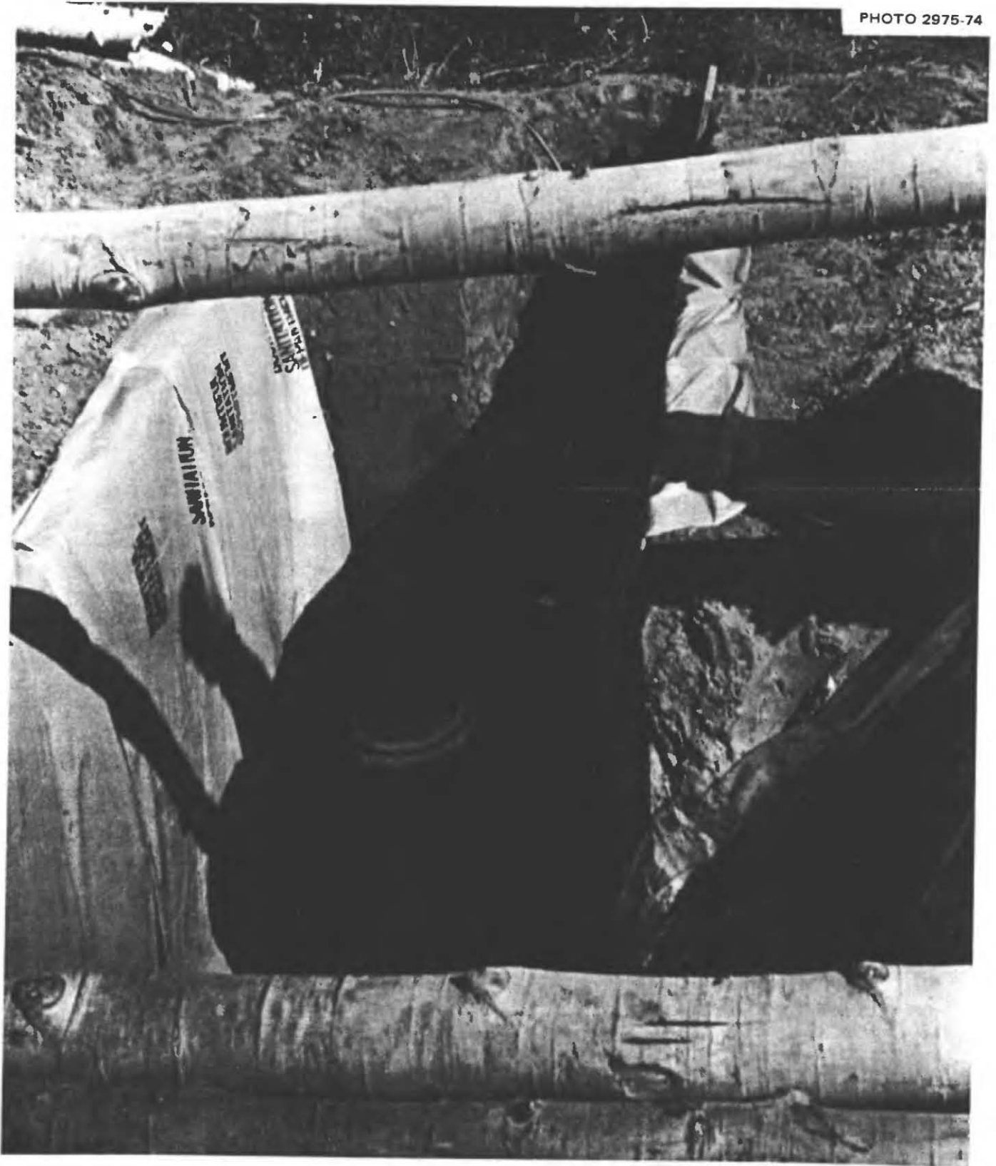
Fig. 4.6. Covering the main trench with 9-ft aspen logs. These logs were 4 to 6 in. in diameter at their small ends – thus being stronger than necessary to support the planned 3 ft of earth cover.
