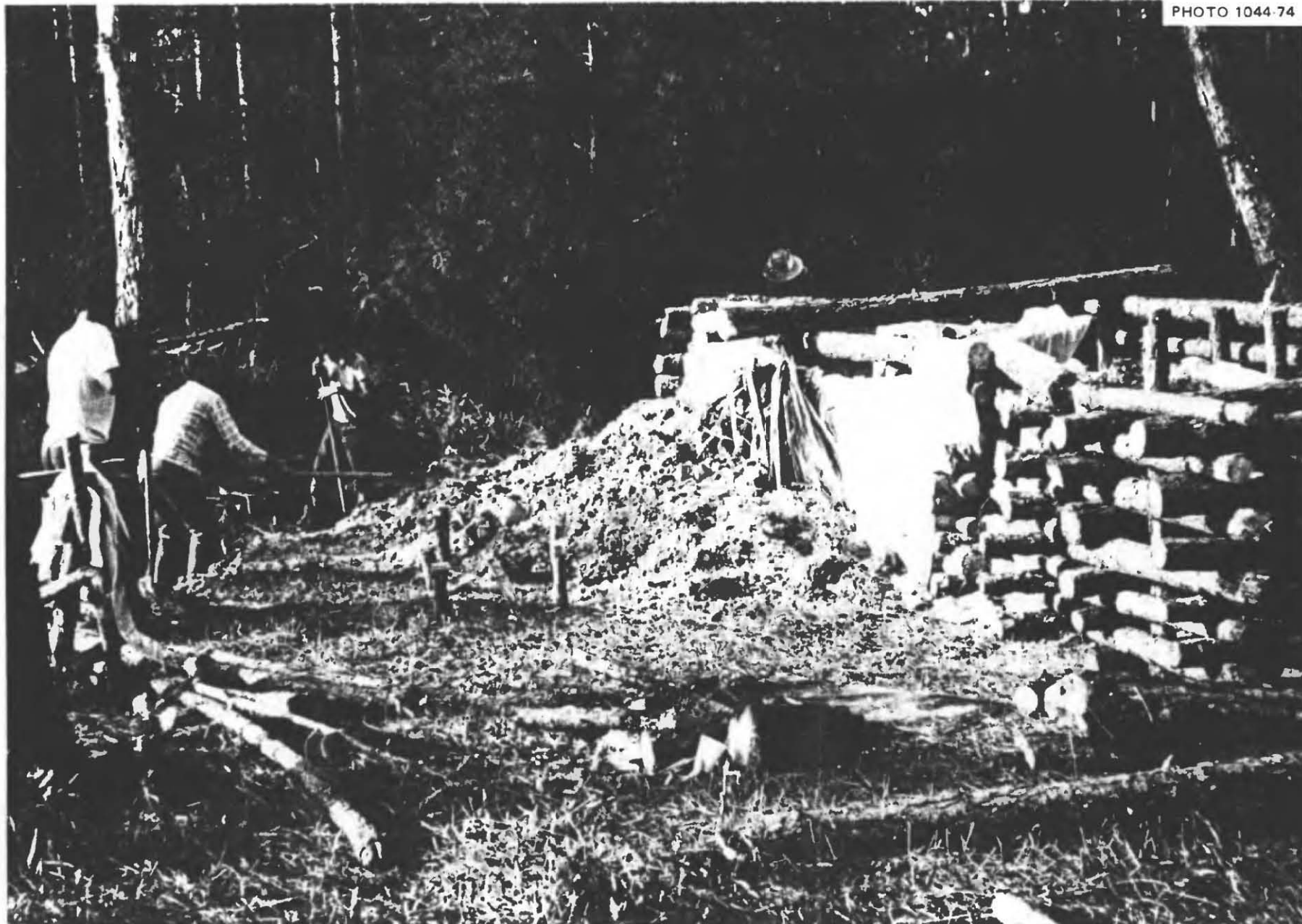
Fig. 5.18. View showing earth being mounded against one of the spaced-pole walls of the shelter. The crib nearest the camera had not yet been lined with a bed sheet, preparatory to filling with earth.
