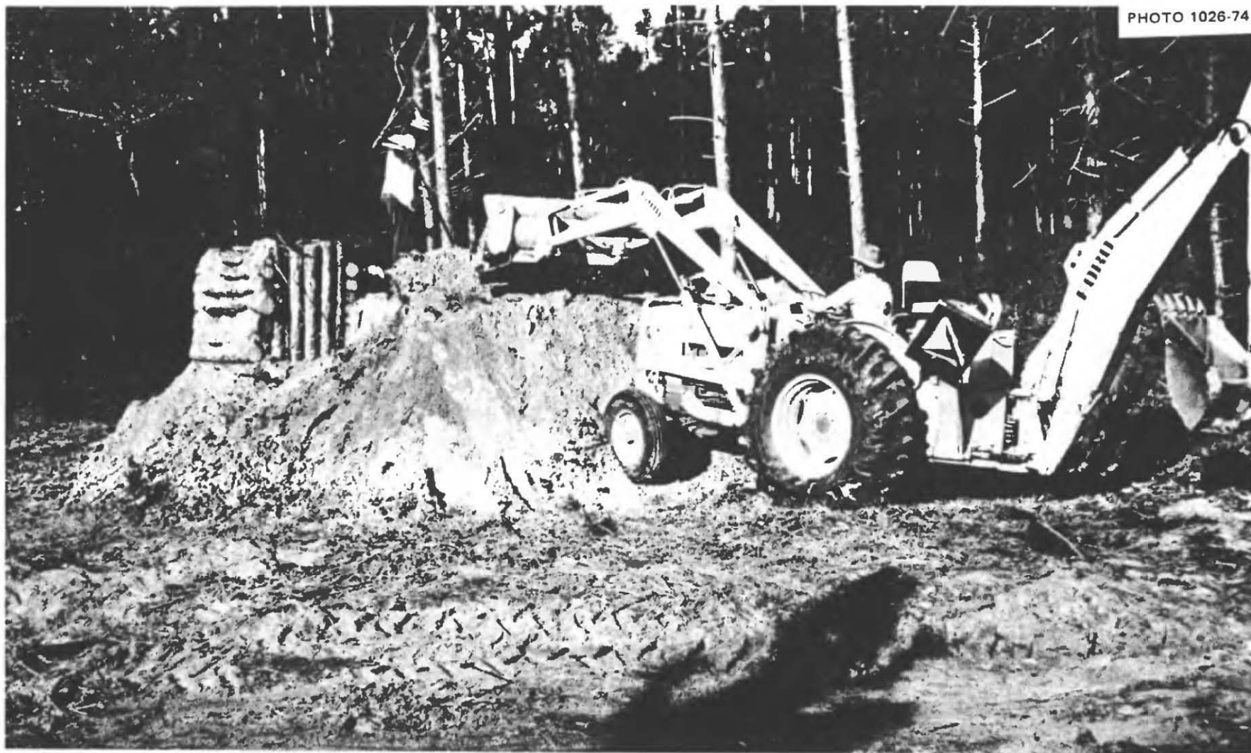
Fig. 5.68. Backhoe covering the unsuccessfully modified Small-Pole Shelter with three rooms built entirely above ground. The backhoe worked for almost 5 hours to place earth on this shelter to a minimum depth of 2 ft, because it could excavate only a little over a foot deep without getting stuck. The backhoe repeatedly had to lift itself out of the mud on both its buckets, although this work was done toward the end of a long dry spell.
