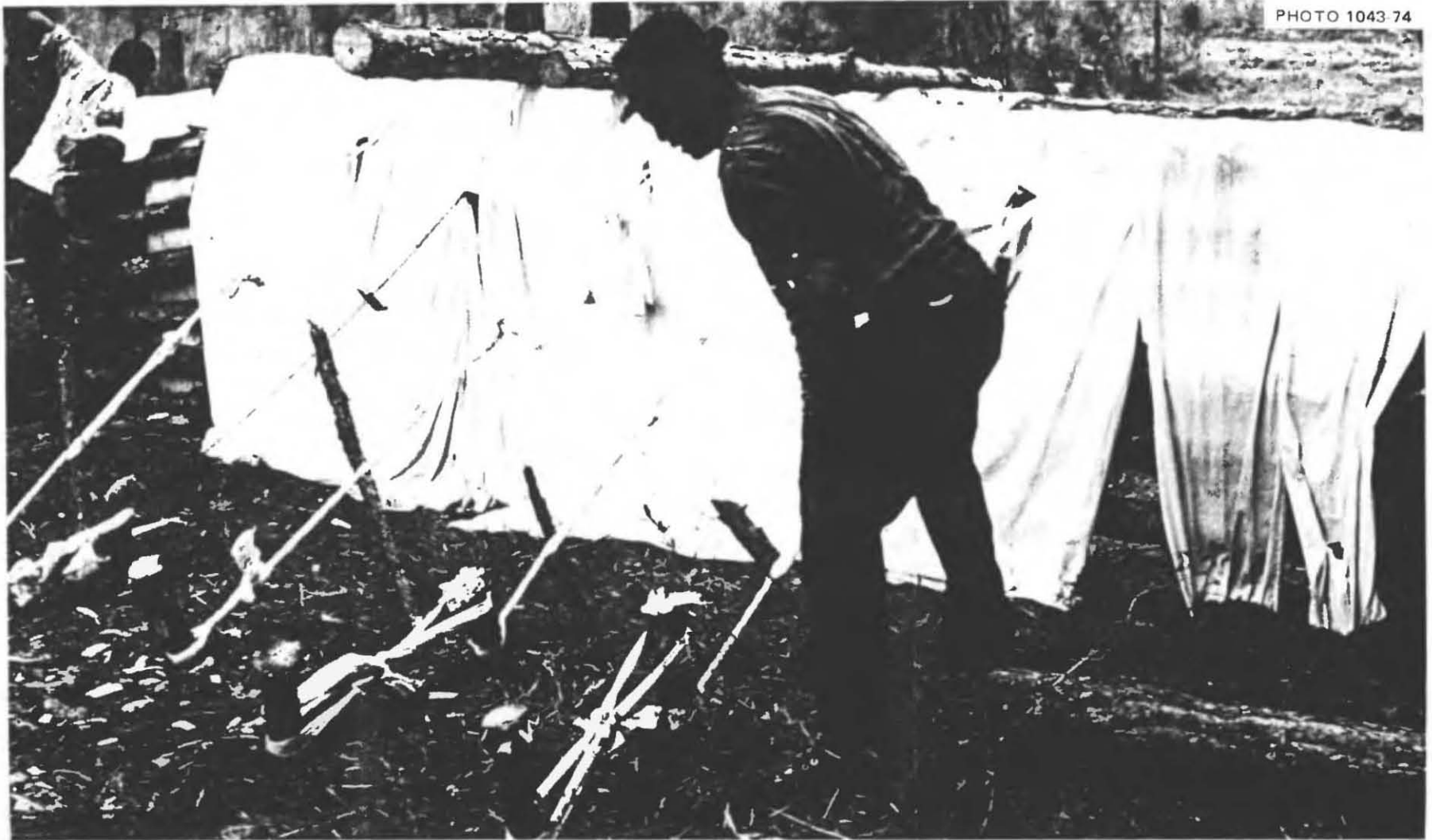
Fig. 5.17. The outside of one of the spaced-pole walls of the shelter room, after it had been readied for mounding earth against it by guying vertical poles against the inside of this wall to stakes driven outside the wall. Note the guy ropes made of foot-wide strips of bed sheets, twisted and pulled tight by the twist-sticks near the inner line of stakes. These twist-sticks are kept from unwinding by being positioned so that their lower ends could be pressed against the ground. Later these guy ropes and sticks were completely covered by the earth mounded against this wall until the 2-ft-wide top layer was about 3 in. higher than the top of the spaced-pole wall. The bed sheets (with the help of earth arching) kept the earth from falling through the spaces between the poles.
