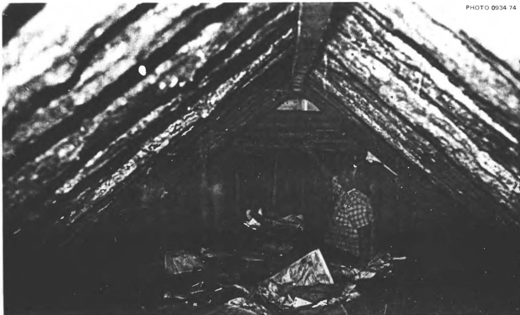
Fig. 5.53. Entrance of the A-Frame Pole Shelter which had a main room 21 ft long and 13 ft wide. If rated a 21-person shelter (as Kearny rated this shelter), this gives each person 13 sq ft of floor space. Both builders and civil defense officials who inspected these shelters agreed that people could get by with 10 sq ft per person of floor space, even though the roof was low and sloping.
