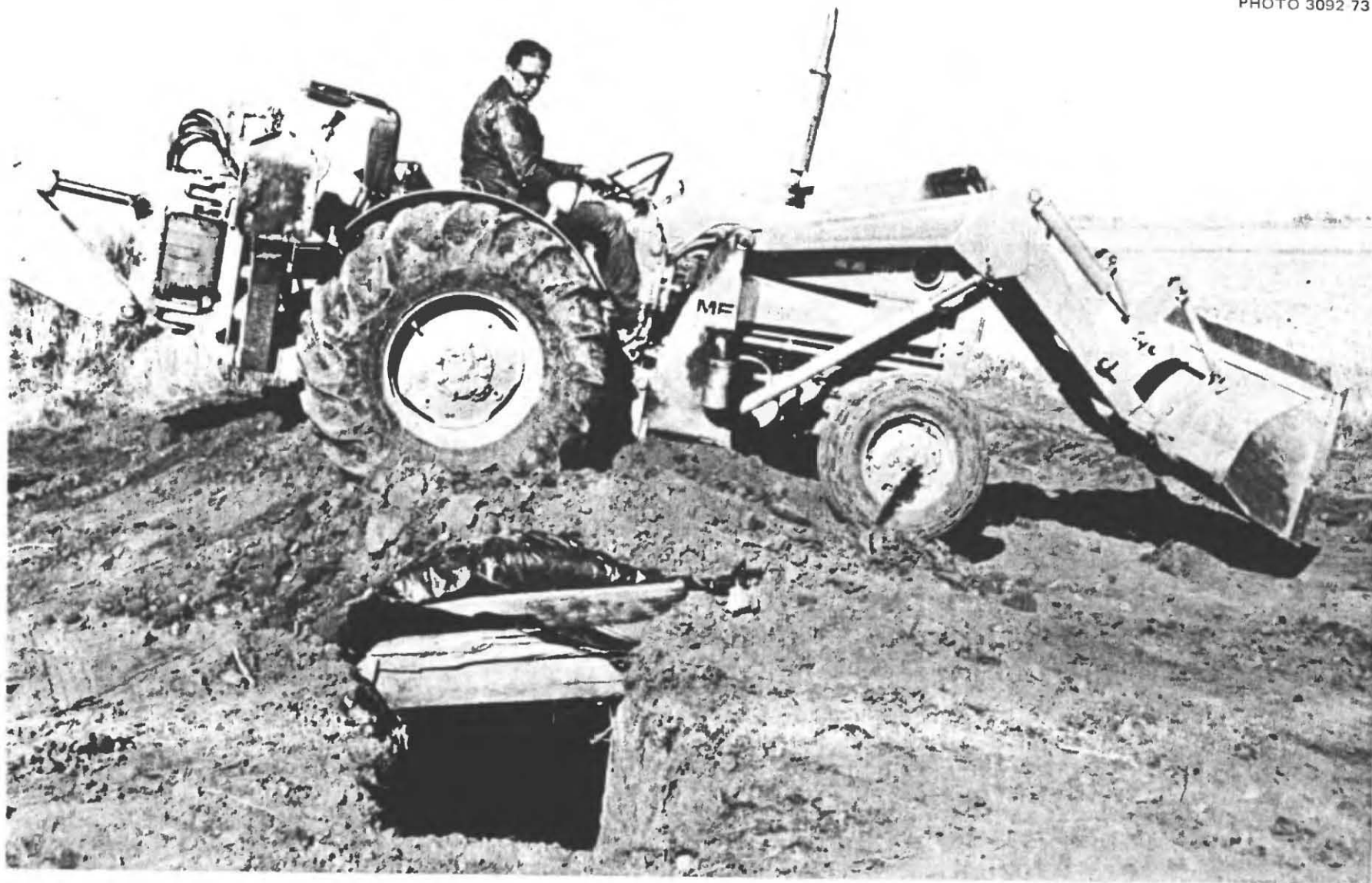
Fig. 3.14. Stressing the Tarp-Roofed Trench Shelter, after the thickness of its earth cover had been reduced to about 3\frac{1}{2} ft, by driving a 6-ton MF-30 backhoe back and forth across it. The downward bow, or sag, of the tarp catenary remained the same (14 in.). Because Kearny wanted to see whether or not the tarp edges in the small earth-filled side trenches had moved, no more of the earth cover was removed preparatory to more severe loading tests. The tarp was unearthed by the backhoe and hand labor; the tarp edges in the small trenches had not been moved, nor had the compacted earth in the two small side trenches been disturbed by the inward pulls on the tarp produced by the loading tests.
