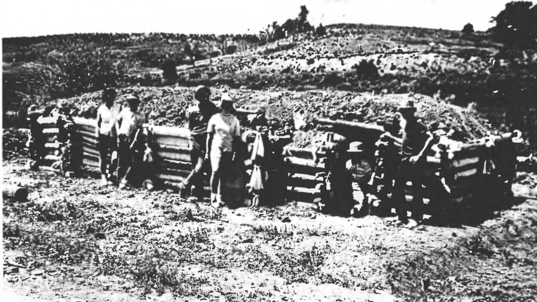
Fig. 5.27. A Crib-Walled Shelter completed in Colorado. This family finished 29 hours and 53 minutes after receiving the building instructions at their suburban-type home about 9 miles away from this site. All six members were at this site, working over 90% of the time, for 10 hours and 13 minutes on May 26th, and for 5 hours and 11 minutes on May 27th. If they had built near a woods and had cut all the poles specified for this shelter, Kearny believes this family could have finished it by working as hard for two full days, 10 or 12 hours each day.
