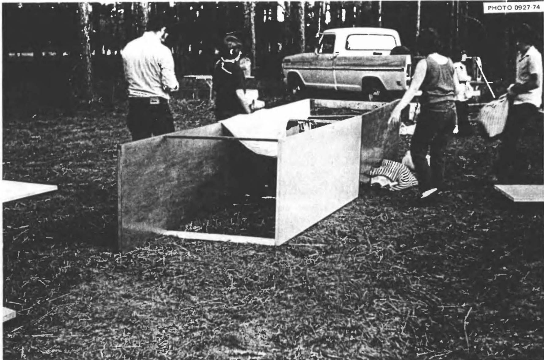
Fig. 5.3. Some of the doors set up as forms around which the earth-filled rolls were built to make the above-ground walls of the 7-person shelter built by this postal clerk, his secretary-wife, their 14- and 12-year-old sons, and their 13- and 9-year-old daughters. Note the cross bracing tacked to the inner edges of the hollow-core doors. These same doors were used for the roof, after the walls made of rolls had been completed.
