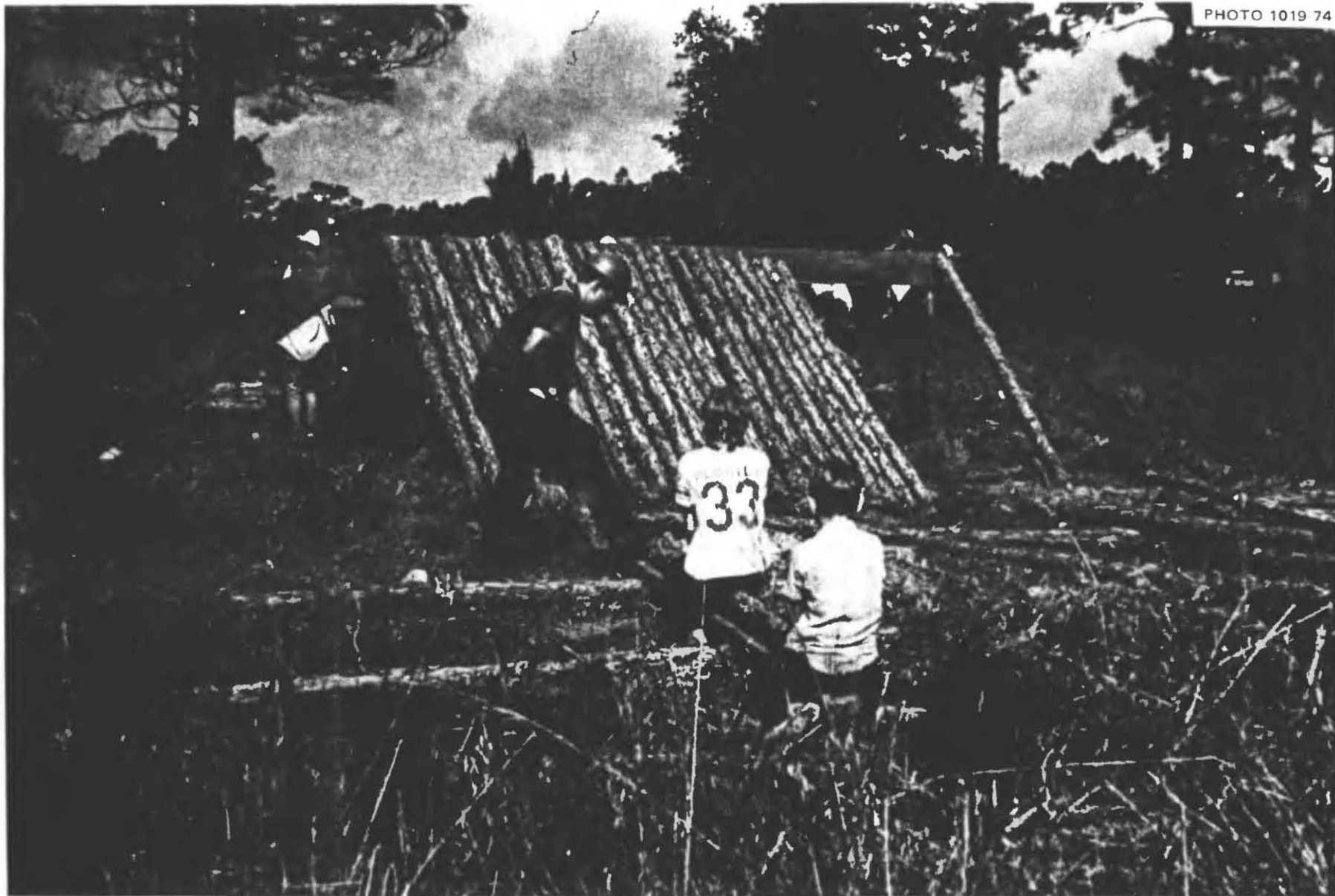
Fig. 5.45. Chain saw operator using a templet to cut an upper end of a wall pole at the specified 54^\circ angle and 9-ft length on its short side. The templet was made from a wide 10-ft board, with one end cut at 54^\circ . A nail was driven 9 ft from the end of this 54^\circ angle; the squared-off base of the pole was placed against this nail.
