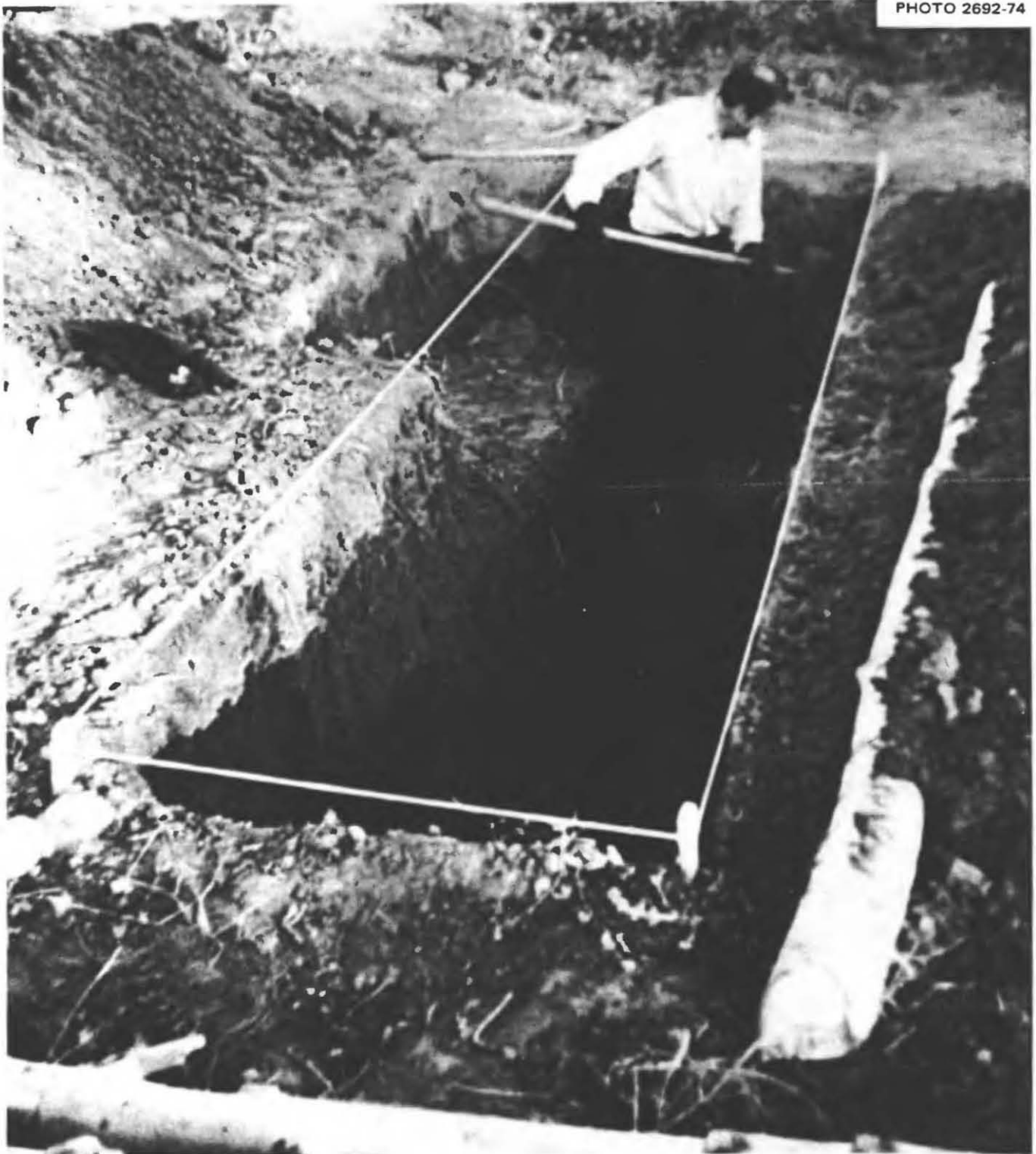
Fig. 4.4. Expanding the shelter room to its full specified width of 3\frac{1}{2} feet, and to its 4\frac{1}{2} -ft depth. This intelligent man made unnecessary work for himself by not following the instructions to cut a 3\frac{1}{2} -ft stick, and then use it repeatedly to be sure the trench was being dug full width.
