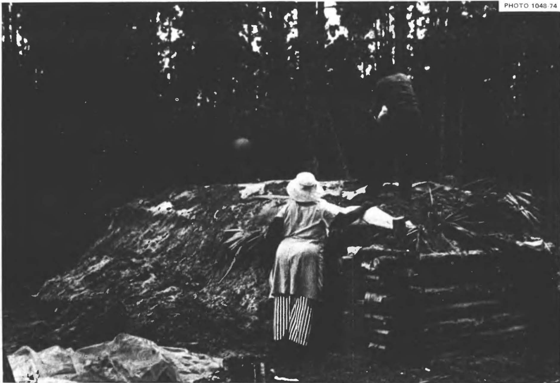
Fig. 5.23. After mounding earth over the shelter roof so that the earth was about 1 ft deep over its centerline, this family made a rainproof "buried roof" out of waterproof material. Since they had part of the north side of their home covered with a big piece of polyethylene film to keep the winter wind from blowing through cracks, they had enough waterproof material to bring with them to the shelter-building site to cover this entire shelter roof.
