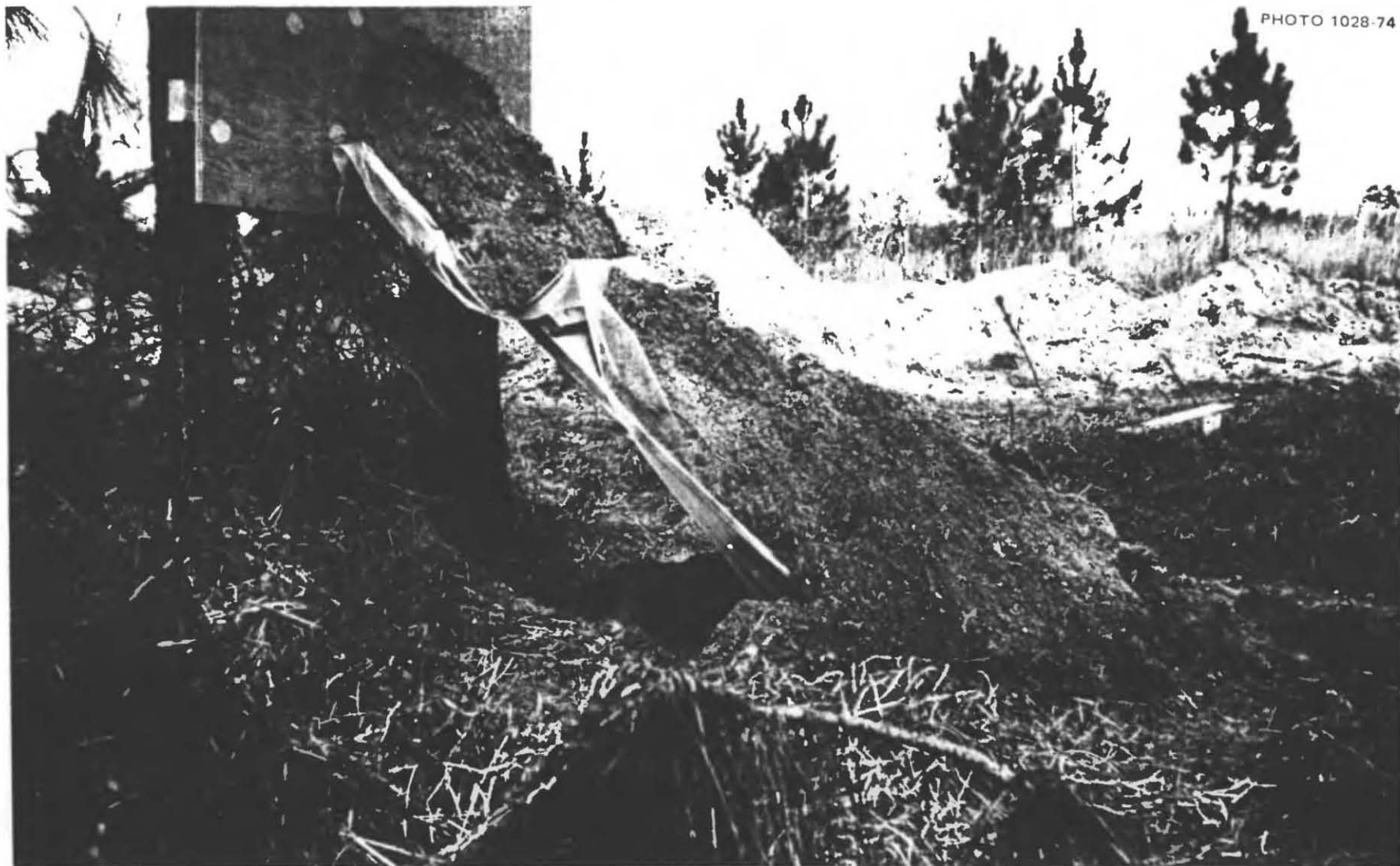
Fig. 5.64. The door was loaded with about half the specified average thickness and weight of earth, due to earth falling off the sides.
