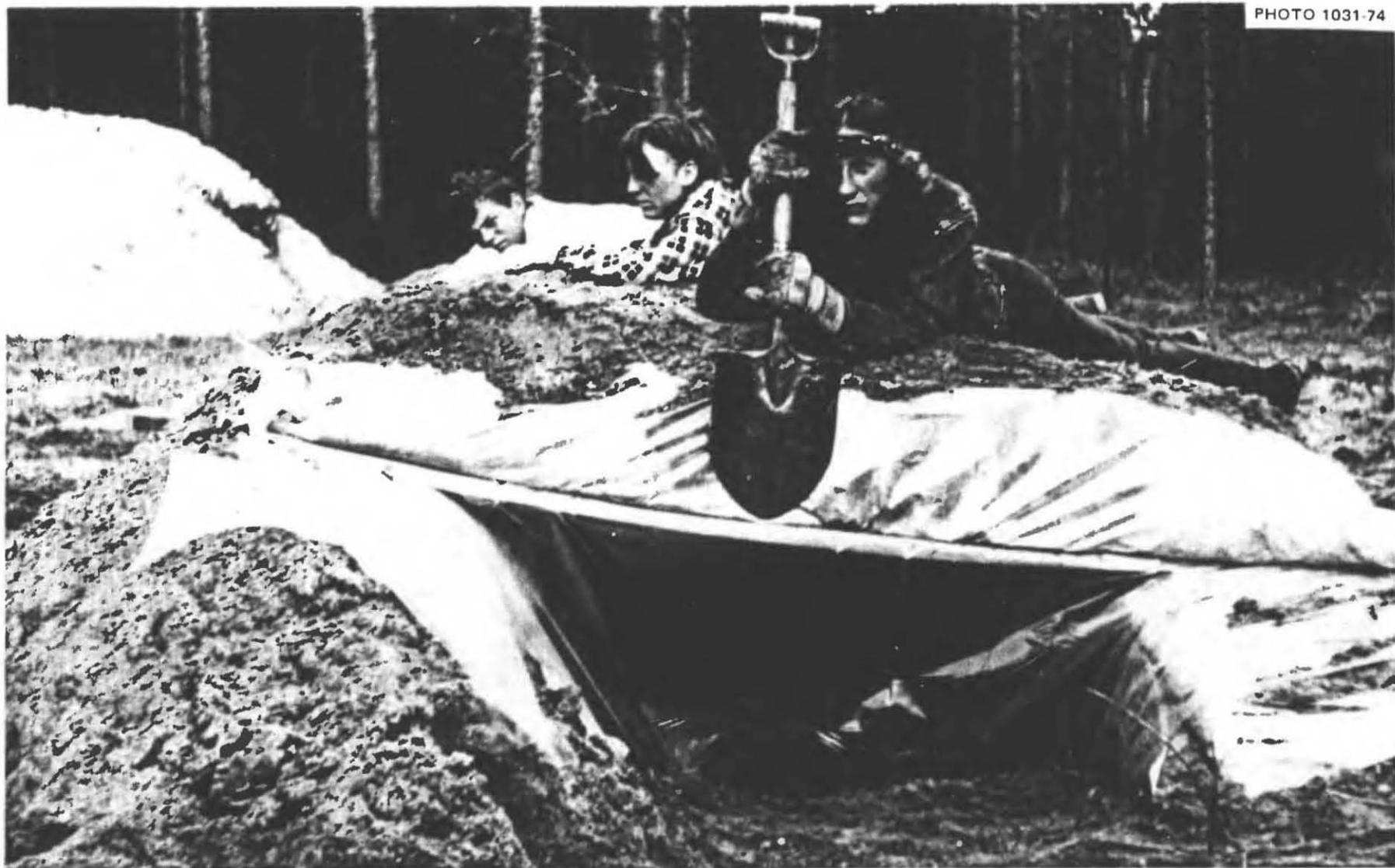
Fig. 5.59. A view of one end of an experimental setup designed to test the strength and dependability of hollow-core doors used to roof an above-ground shelter with vertical walls made of earth-filled rolls, under humid, wet conditions. Two doors that had been painted with two coats of interior-type latex paint were only slightly bowed after being subjected to the pictured loading for almost a month. The doors were protected from moisture by a sheet of 4-mil polyethylene placed directly on them. Note that this roof slopes to the right, so that water will not leak through the plastic.
