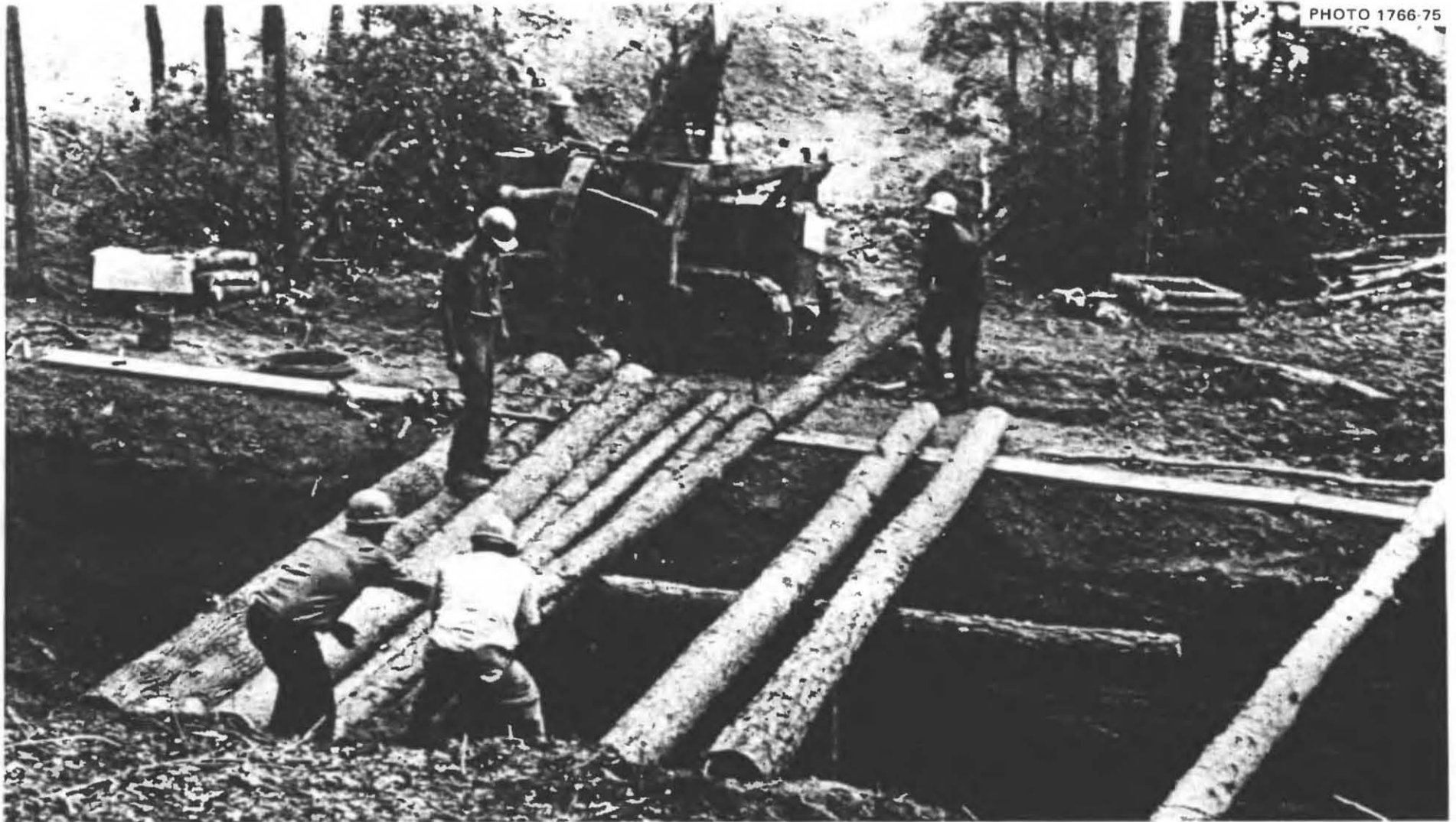
Fig. 7.1. Workmen of a pipeline contractor laying 22-ft logs across a 12-ft-wide bulldozed trench. This trench was bulldozed 7 to 8 ft deep into firm, weathered-in-place Alabama clay. The sides of the trench were vertical.
