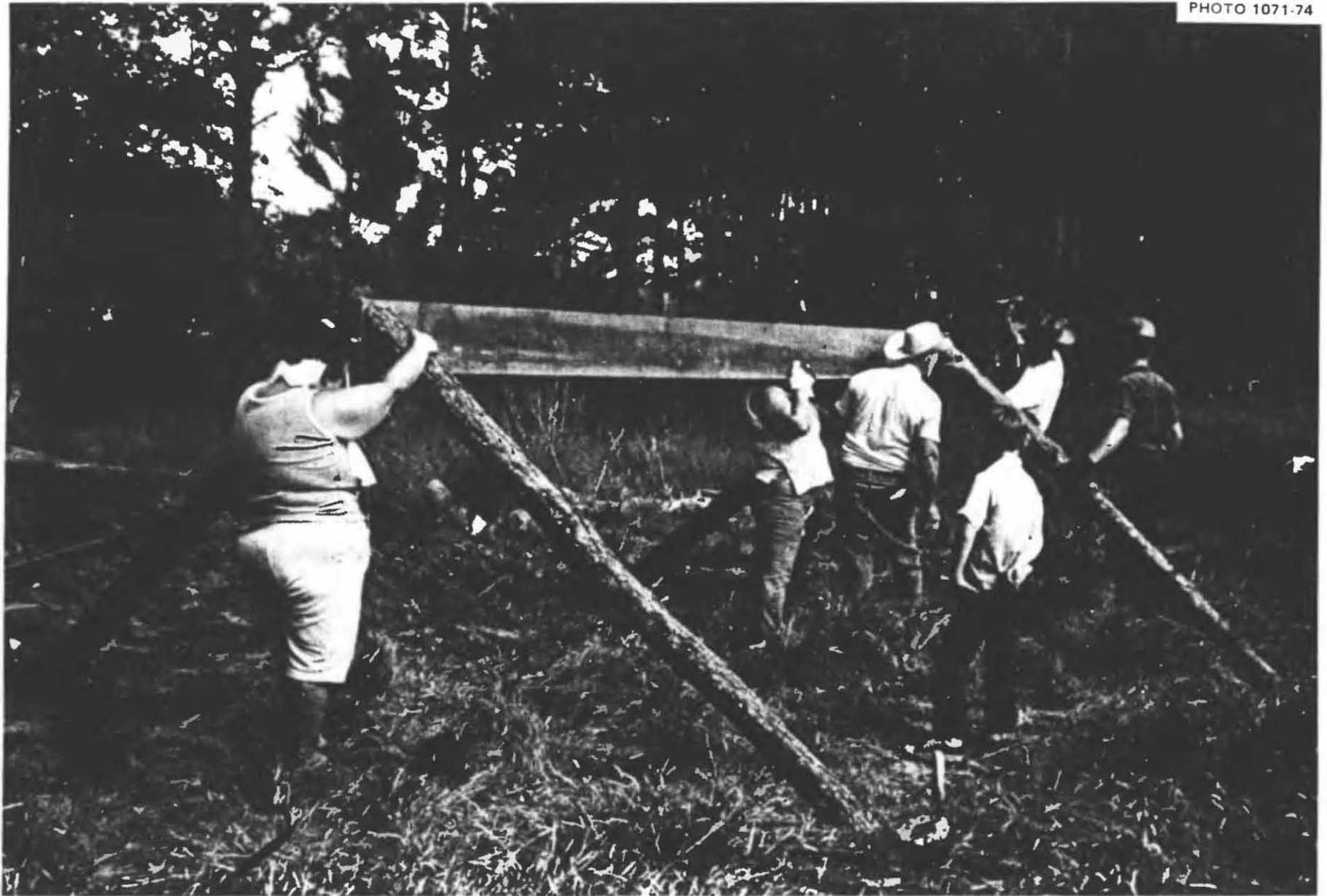
Fig. 5.44. Erecting a 16-ft-long section of the ridge board that later was extended to a 21-ft length. These decidedly competent rural people were so overconfident of their building abilities that they failed to read the instructions carefully. As a result, they made several errors that they had to correct. One of these errors was initially using a 5-in.-wide board for the first part of the ridge board; they found that the upper ends of some of the wall poles would not fit properly against a board so narrow.
