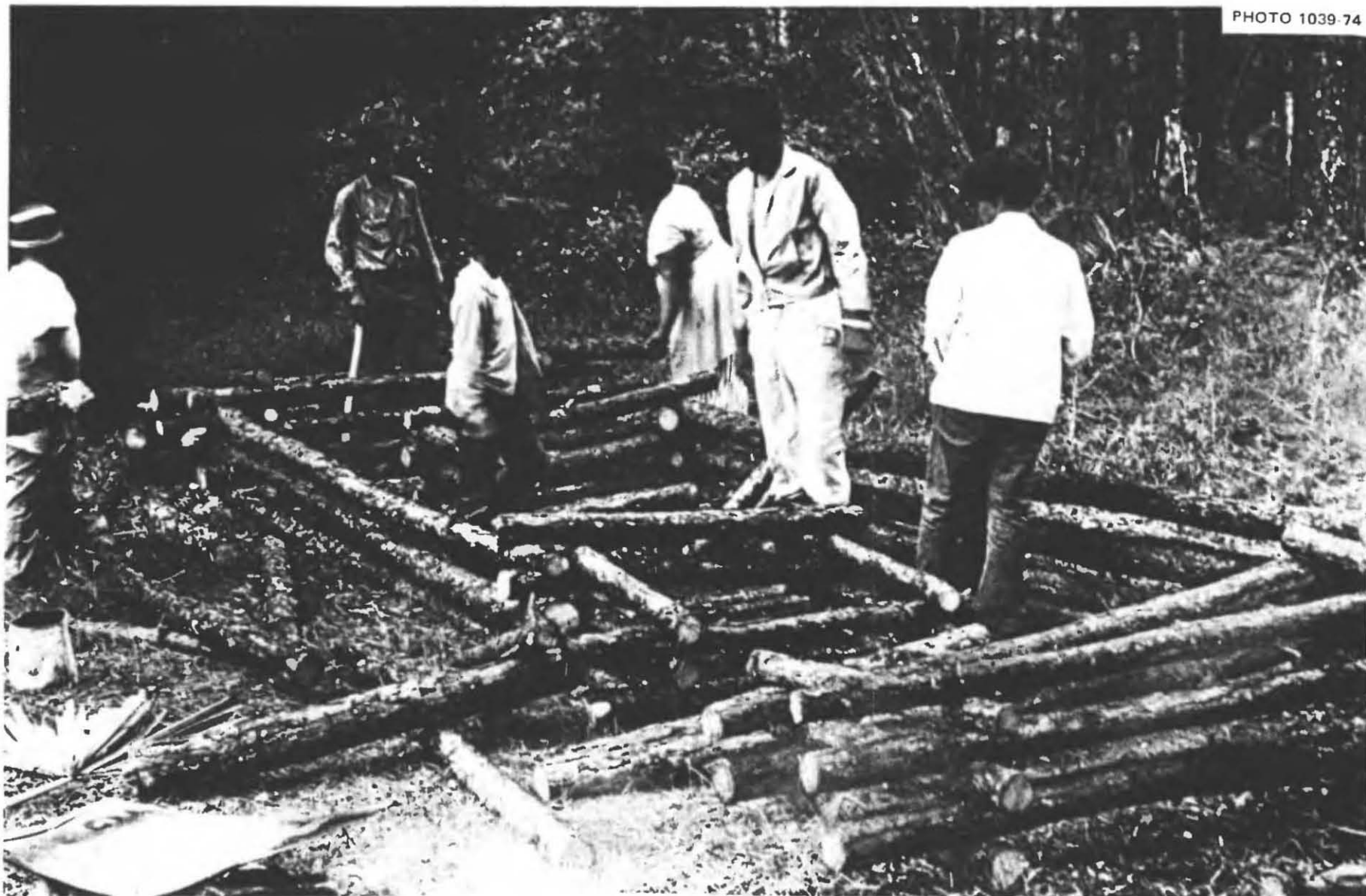
Fig. 5.16. Building the cribs forming the entrances and ends of this shelter, and also making the connecting spaced-pole walls of the main room. This family of 6 consisted of a father, aged 55, who is a painter and odd-job handyman; a mother, aged 50, who is a school custodian; a son and daughter, both 16; and two small but strong sons, aged 13 and 11.
