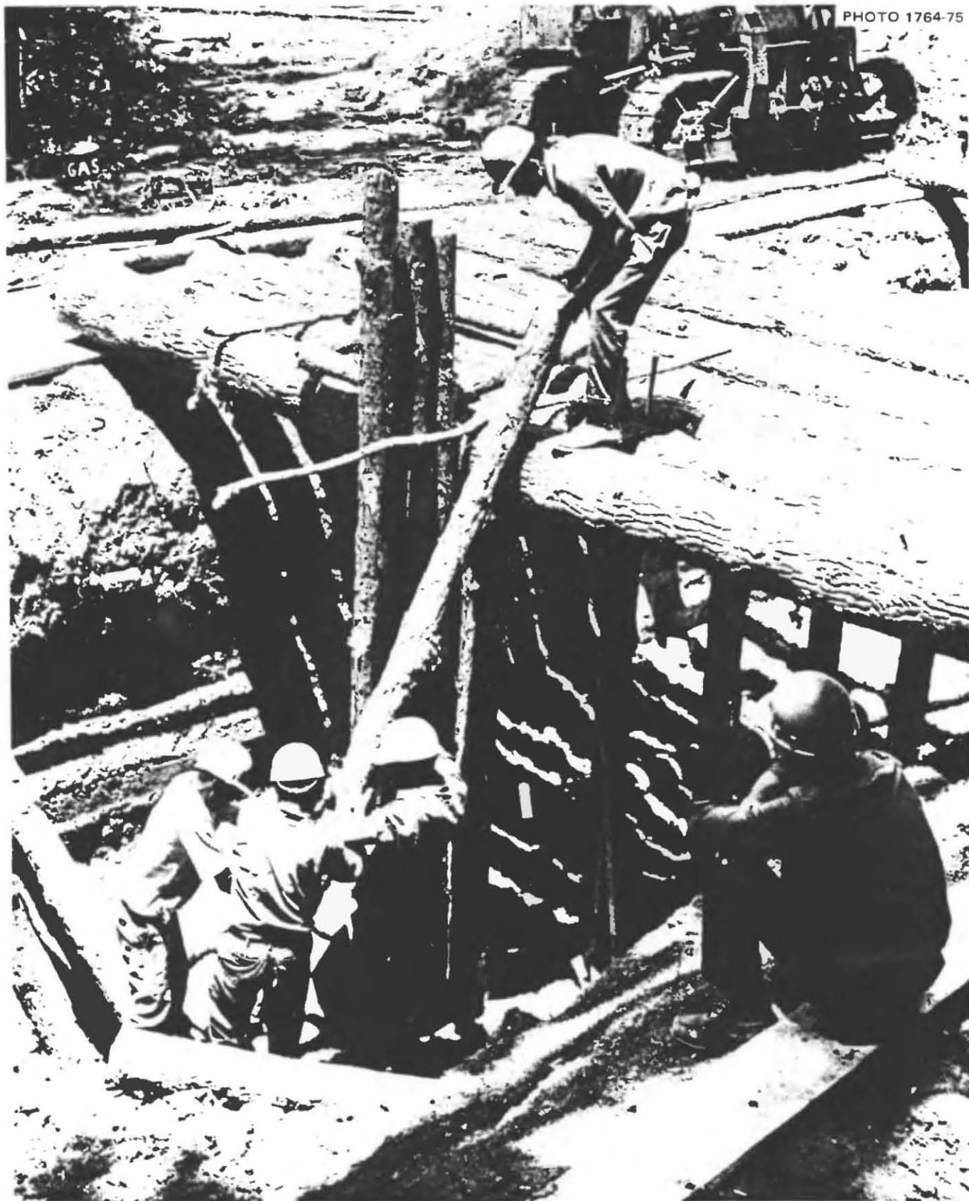
Fig. 7.2. Starting to erect one side of an entryway, after all of the 22-ft roofing logs had been positioned. A vertical entryway was placed at each end of the 12 × 42 ft shelter room.
