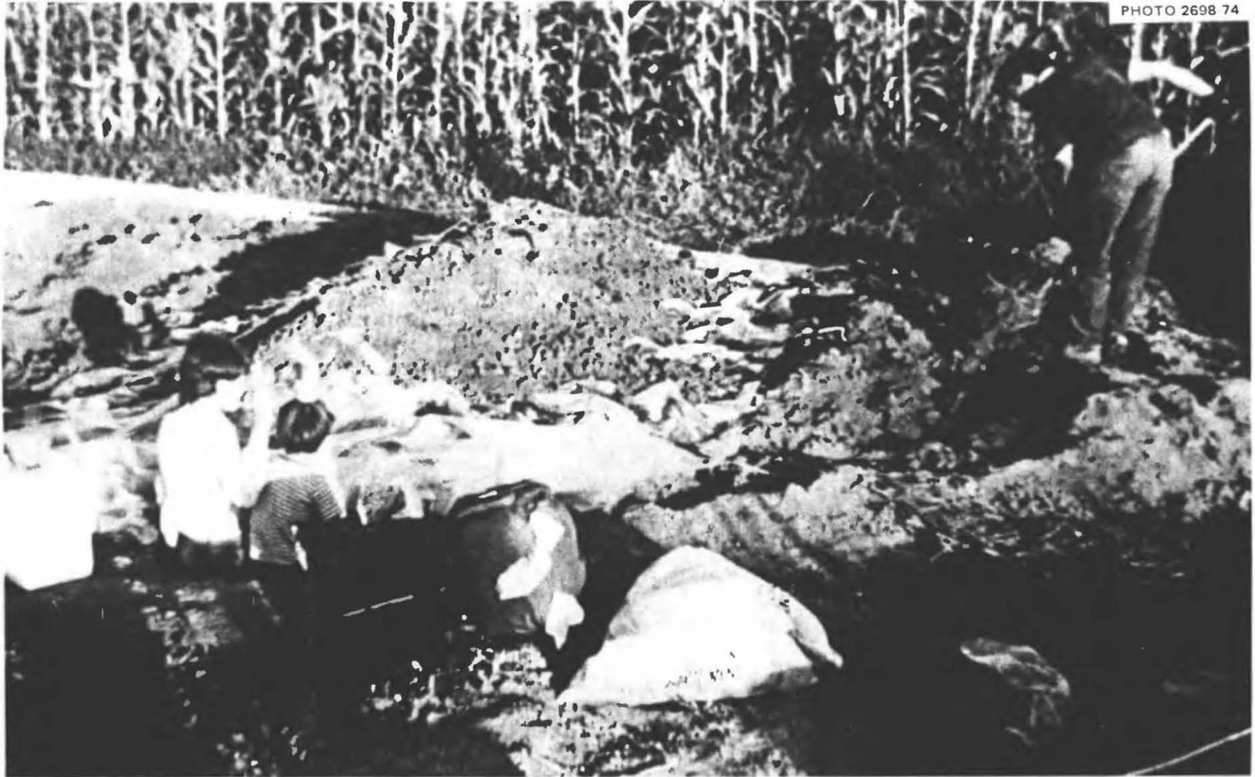
Fig. 4.9. Shoveling earth onto the "buried roof" made of a large piece of 4-mil polyethylene. After earth had been mounded onto the roof logs until it was about 18 in. deep along the centerline, the polyethylene sheet was spread over the entire roof area.
