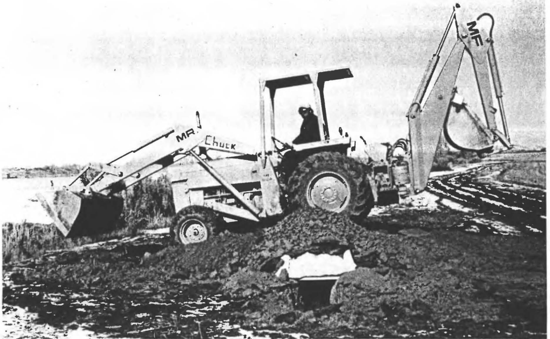
Fig. 3.5. In order to break the roofing doors, the backhoe removed all but about a 2-ft thickness of the earth covering. Then the 8-ton backhoe was driven over the shelter; this compacted the earth under the wheels (reducing its thickness to 21\frac{1}{2} in.) and suddenly broke the \frac{1}{8} -inch mahogany veneer on the lower sides of two doors. But the \frac{1}{8} -in. veneer on the upper sides of the doors did not break!
