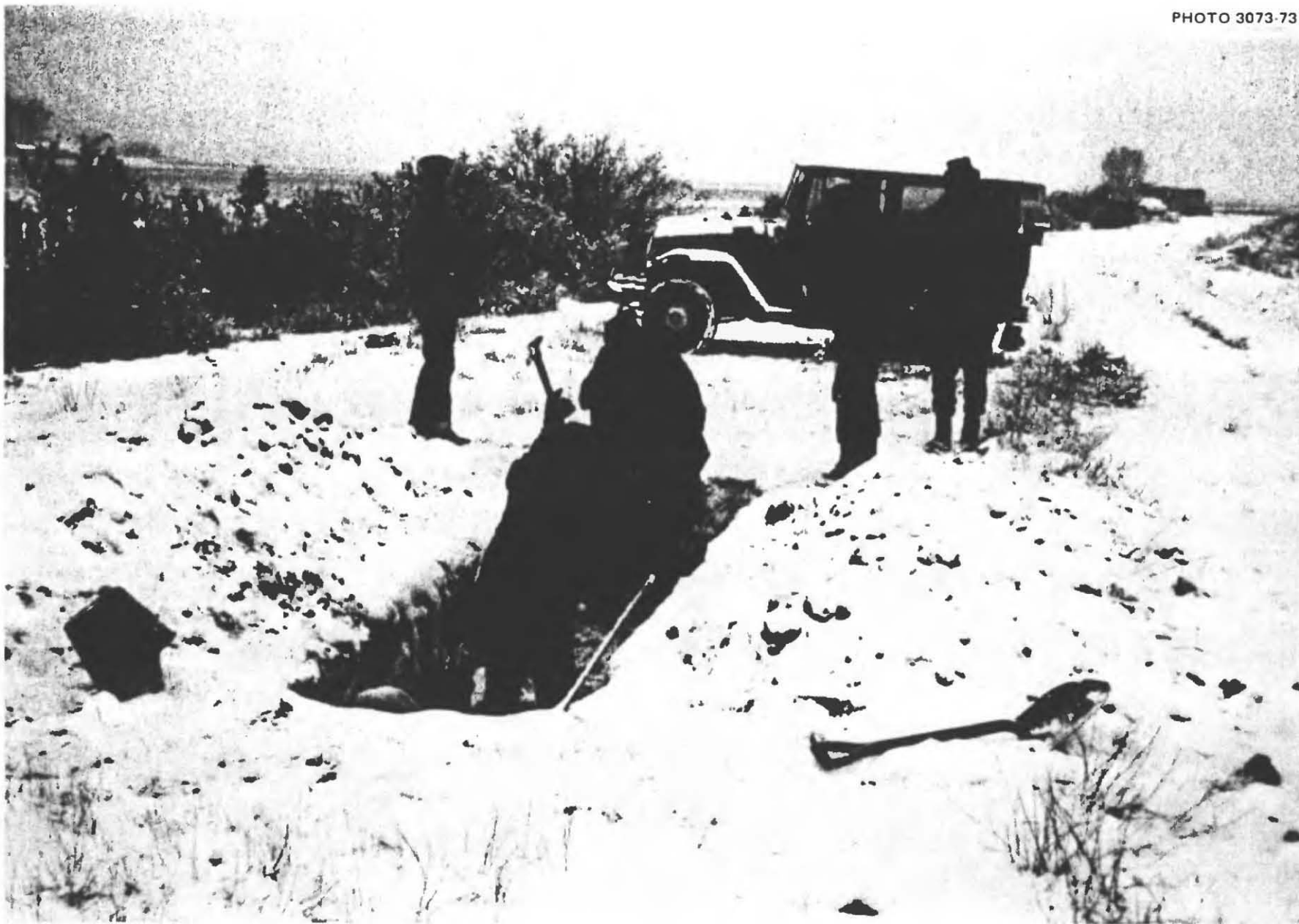
Fig. 2.6. Starting work at 7:33 AM on the second day, sore of muscle and low in spirits. It was snowing intermittently, at 25° F. All six workers were on the job the second day until completion of their shelter.
